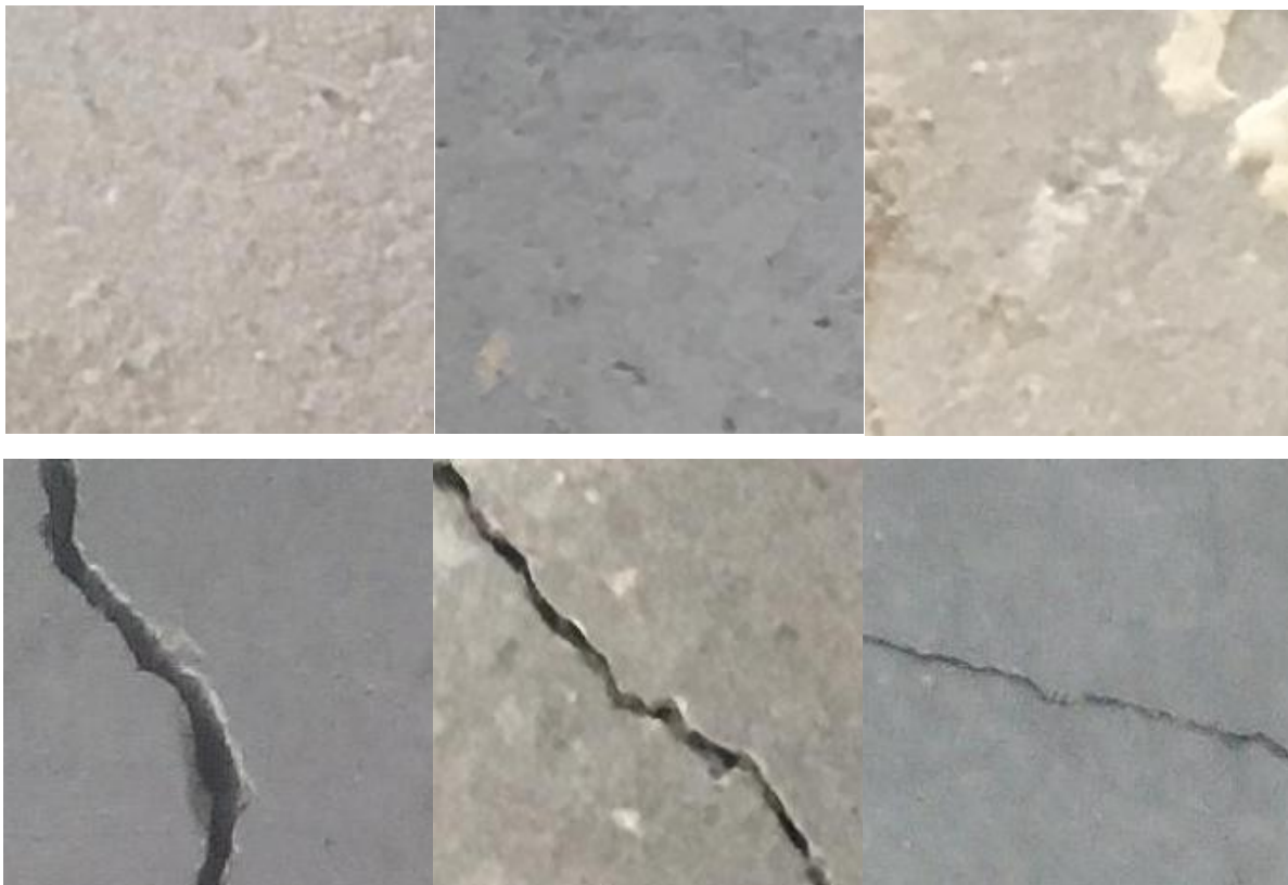
Figure 1. Examples of images in dataset. first row: normal surface, second row: cracked surface
